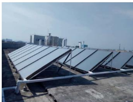
Solar heating system of Jiangmen Factory
